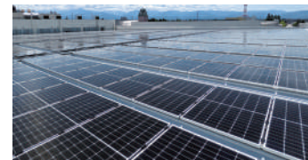
The solar power generation system on the roof of the No. 3 Robot Factory
